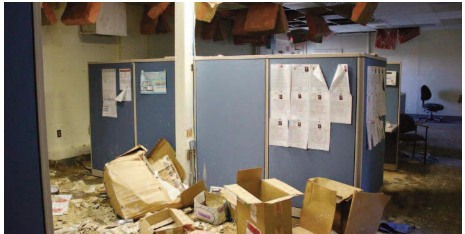
Interior damage caused by Hurricane Florence is shown at the Provost Marshall Office facility at Marine Corps Air Station Cherry Point in November. The building is incapable of being occupied. Roughly 800 buildings at Marine Corps Base Camp Lejeune, Marine Corps Air Station New River and Marine Corps Air Station Cherry Point were damaged during the storm. (Photo by Allie Erenbaum, originally published in Camp Lejeune Globe in January, 2019)
